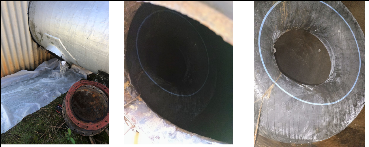
With headgate closed leakage needed to be blocked to stop flows from getting to the powerhouse. Sebastian came up with an idea to insert an inner tube through the access hatch below the Rotax and inflate along with opening the Rotax house drain valve allowing flows to be monitored through S76A weir.
