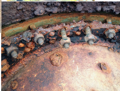
These cap screws are what holds the seat in place and obviously aren't doing their job.
